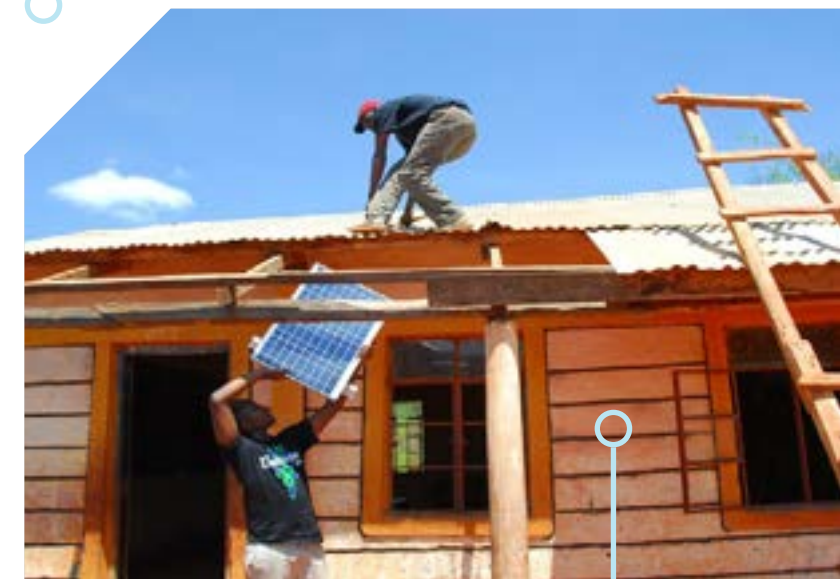
IEEE's Kenya student branch installs solar panels at the isolated Kasiluni Primary School, the only institution of its kind within a 25-kilometer radius. The school serves 600 pupils in six grade levels.
